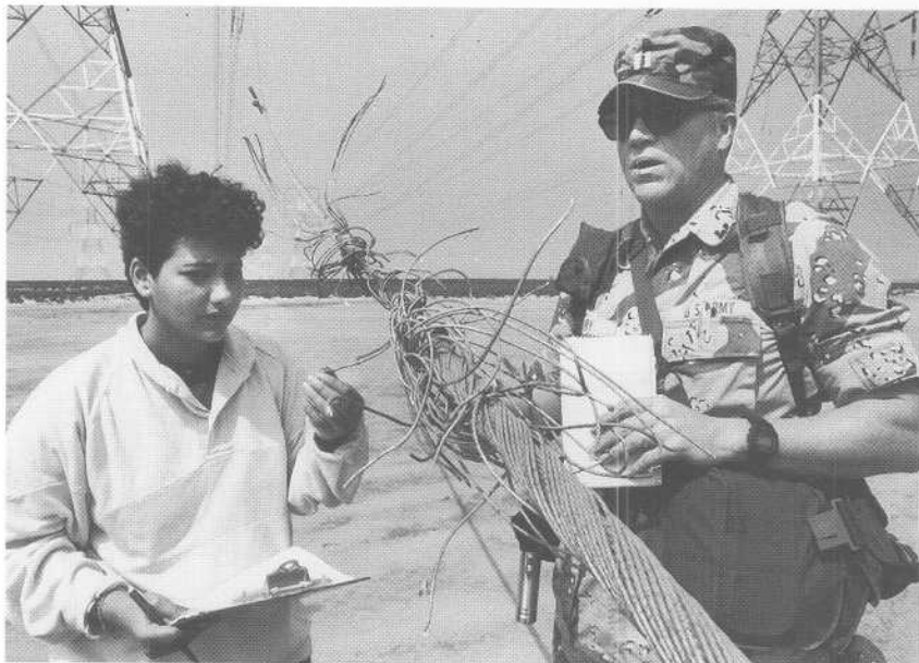
Kuwaiti volunteer Eman Al-Qurba and Corps Capt. Bob Irby assess damage to power lines.
